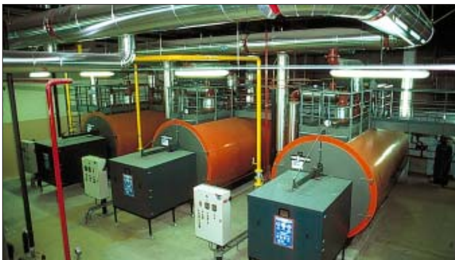
Chaufferie centrale, place Paul Verlaine.
